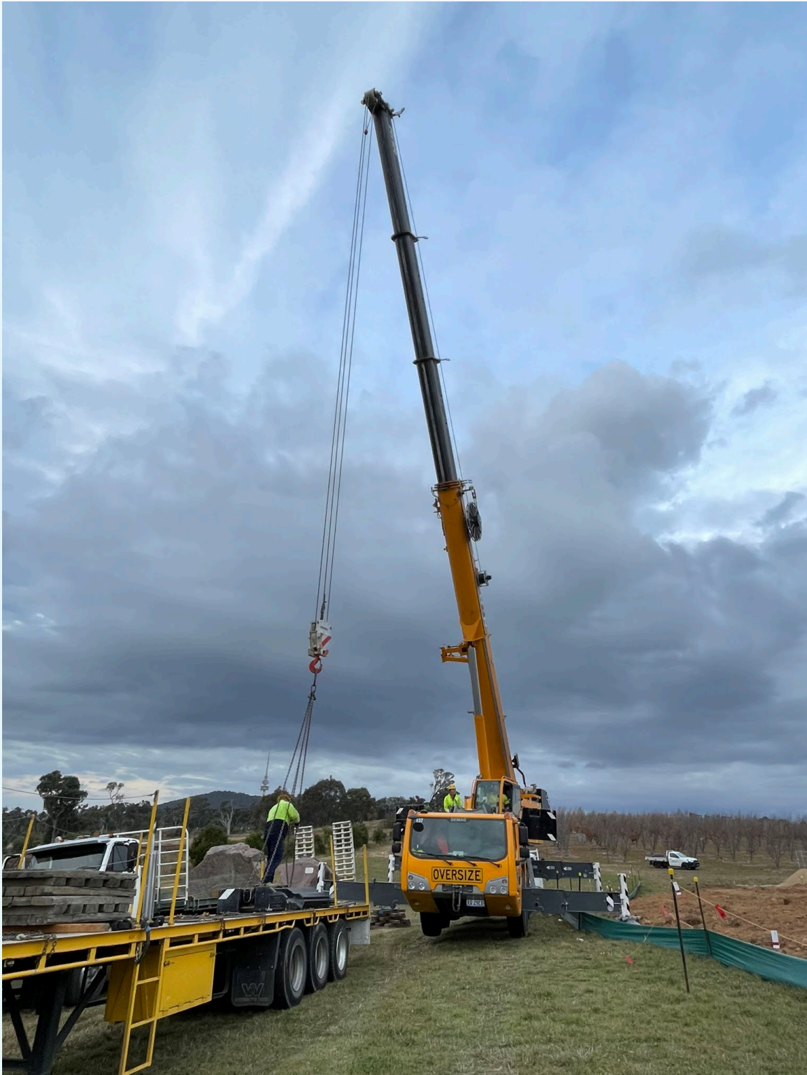
A big rock needs a BIG crane! Preparing to transfer the last of the Federation Rocks to their new home. Image courtesy M. Cooper.
