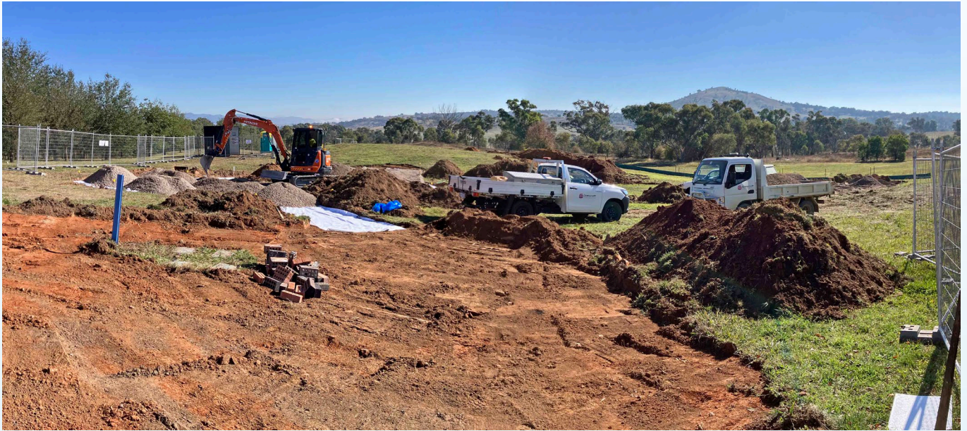
Excavation work at the National Rock Garden in May 2024. Geotextile fabric is being rolled out and covered with a gravel subbase. Image courtesy B. Pillans.
